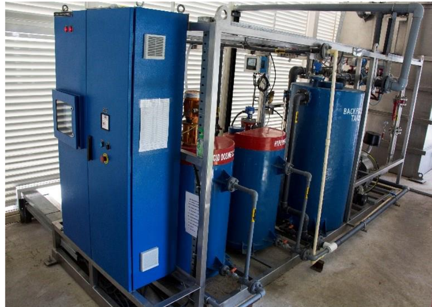
Sewage treatment plant with MBR technology
